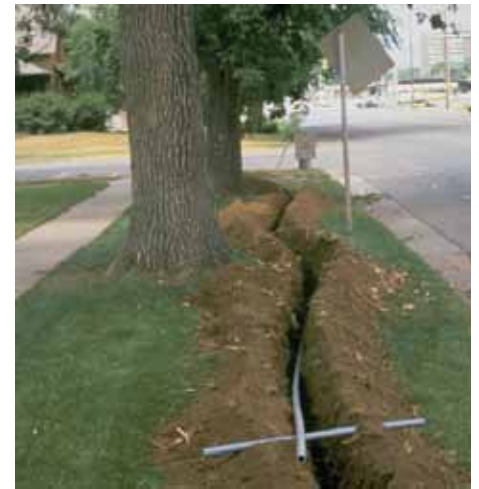
Figure 5: Trenching near trees can severely damage root systems.
