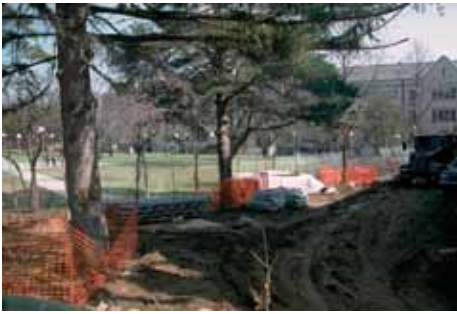
Figure 6: Construction vehicles can damage the existing soil structure by compressing soil particles.
