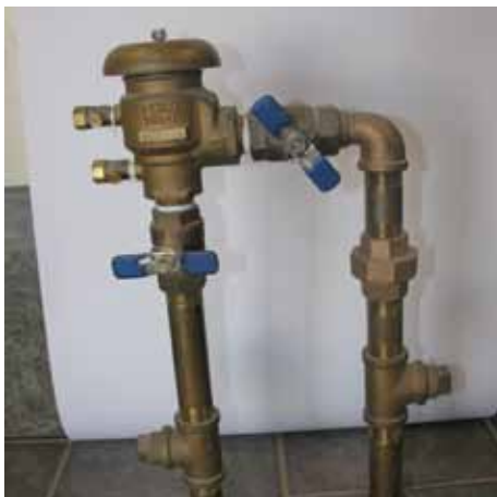
Figure 3a: Left Photo – Pressure vacuum backflow device (PVB).
