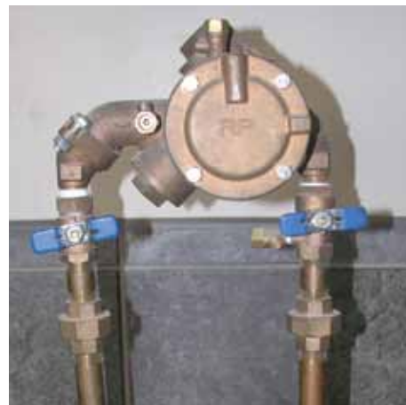
Figure 3b: Right Photo – Reduced Pressure back flow device (RP). Blue handles designate isolation ball valves. Note blowout fittings (tees with threaded plugs) on either side of the device.
