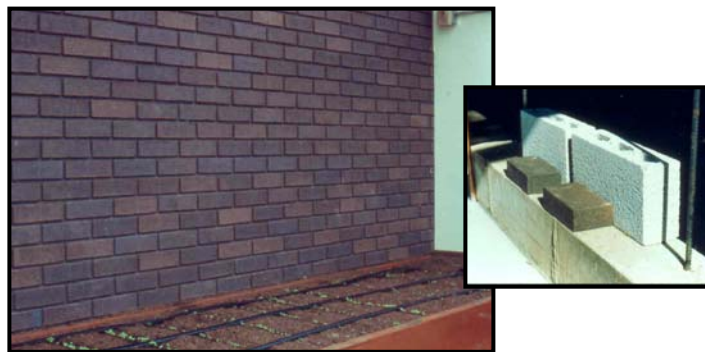
Figure 1. Brick storage wall in passive solar hobby greenhouse – Thermal storage mass is a wall made with two layers of brick filled with concrete. In this well-built structure, nighttime temperatures dropped to 35° with no supplemental heat when outside temperatures dropped to -17°. Note young crops in raised-bed style garden with
