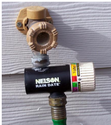
Figure 2. Single zone controllers connect to the hose line. Left: This style is manually turned on and automatically turns off after the set number of minutes. Right: This style turns water off and on at the day and time intervals set by the gardener.
