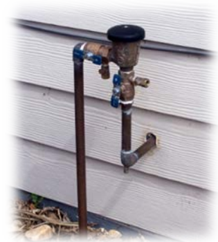
Figure 2. Required by local building codes, backflow prevention devices are typically located where the line comes outside from the house.
