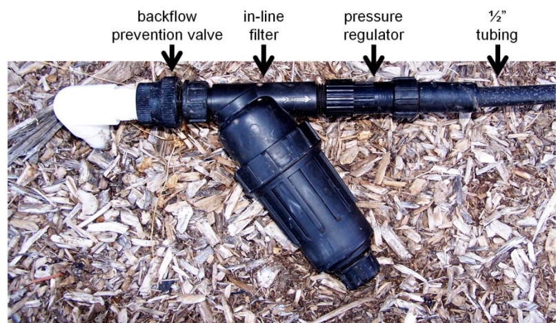
Figure 9. In-line filter and pressure regulator going to drip line poly tubing.
