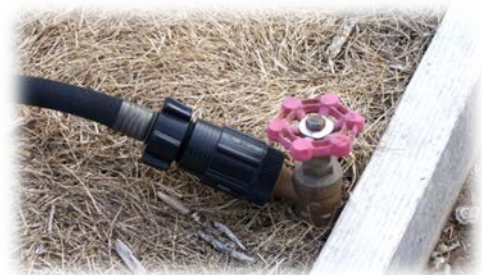
Figure 11. Tap, pressure regulator (with hose connections) and half-inch drip hose in raised bed garden.
