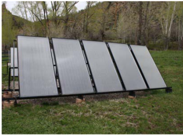
Ground Mount Solar
